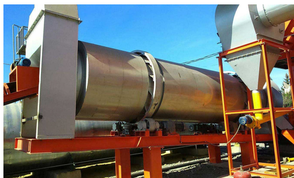
3. Dryer & Burning System
