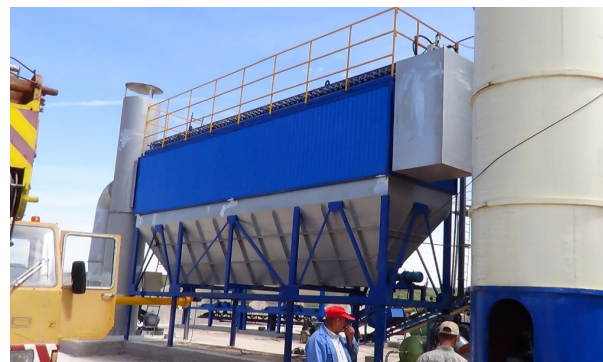
2. Dust Collector System
